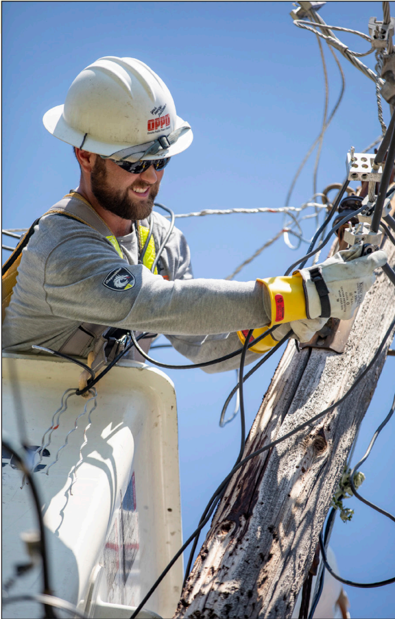
Above and top: Crews work to restore power after the July 31 windstorm that caused more than 221,000 customers to lose power.
