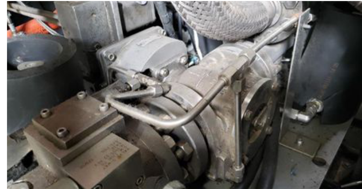
Natural Gas Valve
