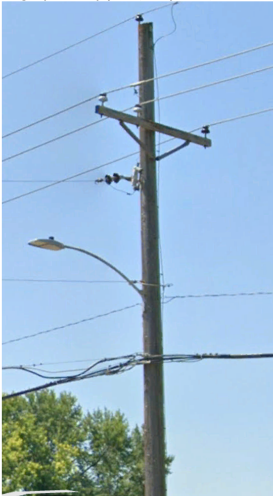
Single-phase tap pole (acceptable)
