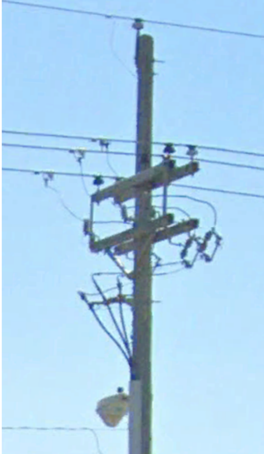
Three Phase Cable Terminal Pole
