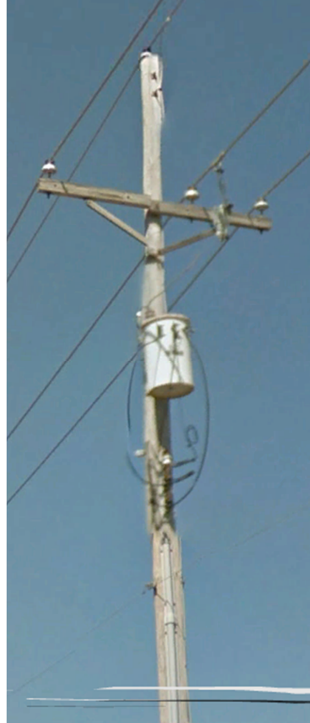
Single Phase Truck Accessible Transformer Pole
