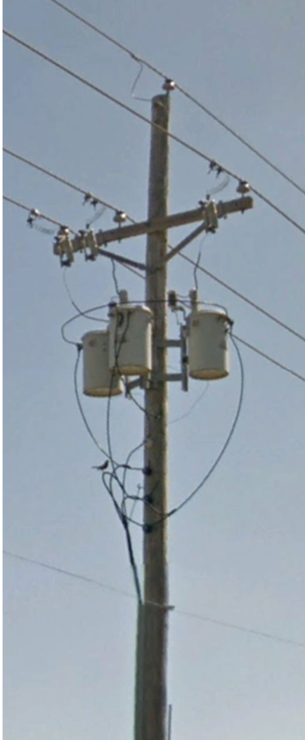
Three Phase Truck Accessible Transformer Pole
