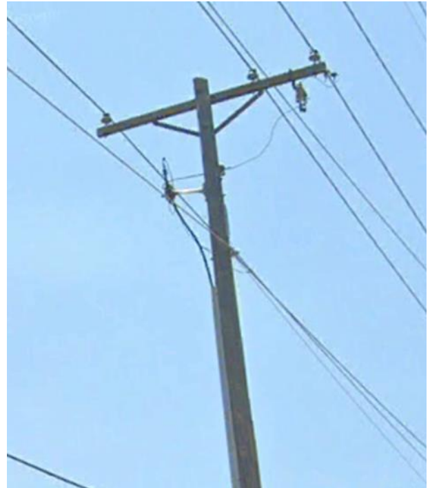
1-Phase Cable Terminal Pole:
