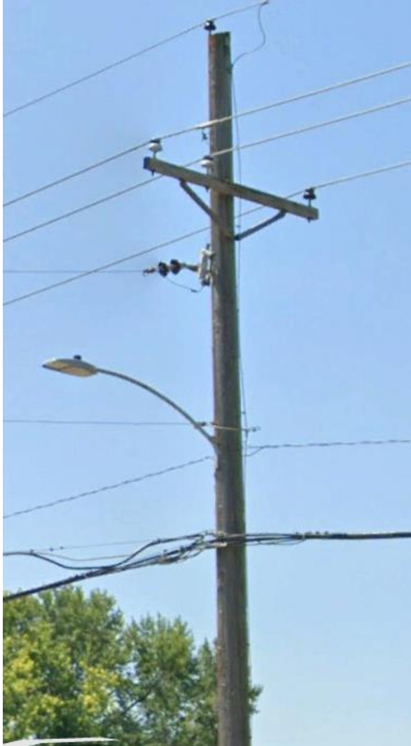
Single-phase tap pole (acceptable)
