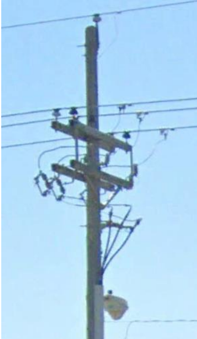
3-Phase Cable Terminal Pole:
