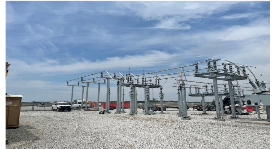
OPPD Substation – Bus Extension to AES Collector Substation
