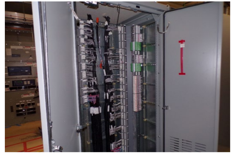
Distributed Control System Cabinet
