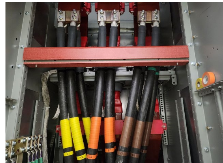
13.8kV Cable Terminations
