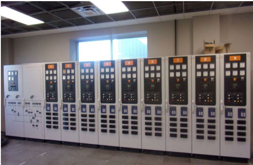
Wartsila Cabinets in Control Room
