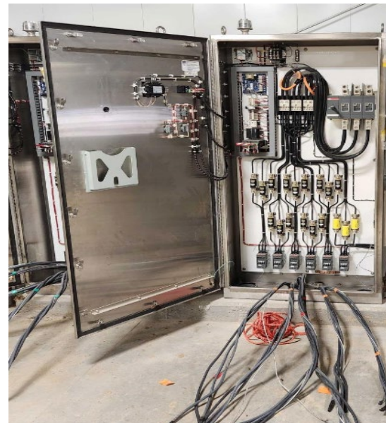
Control Panel Terminations in Fuel Building
