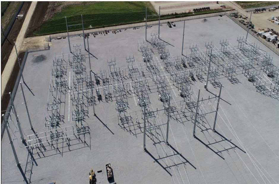
Facing South – Substation Aerial
