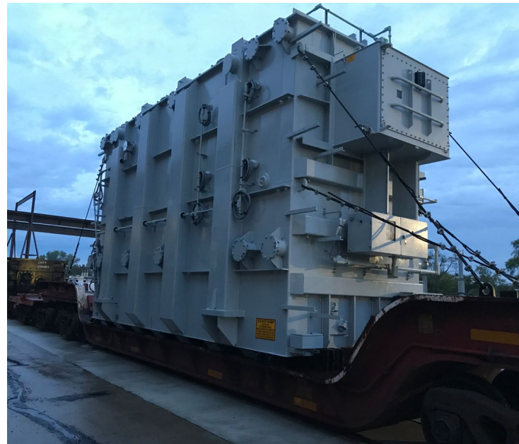
Generator Step-Up Transformer
