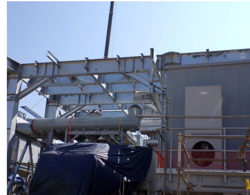
Facing East - Unit #1 Isophase Staging
