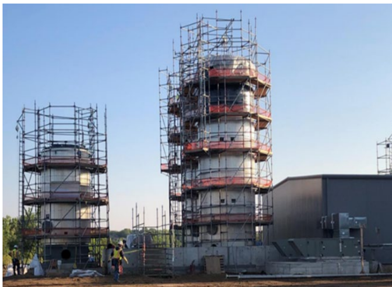
Facing North – Service Water/Urea Tanks Insulation
