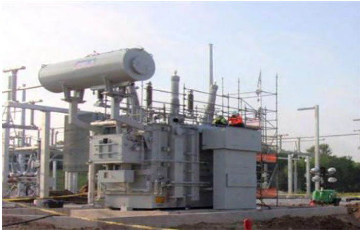
Facing Southeast - Generator Step-Up Transformer
