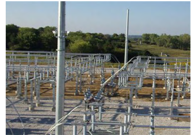
Facing South - Substation
