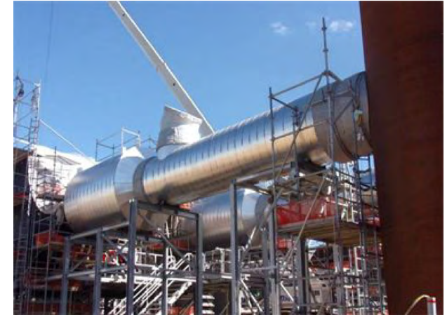
Engine Horizontal Ductwork/Insulation to Stack
