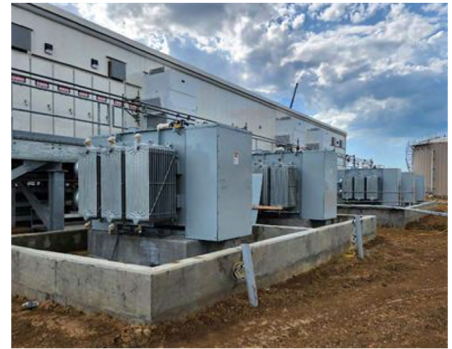
Station Service Transformers on Foundation
