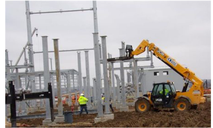
Facing West – Substation H-Frame & Switch Placement
