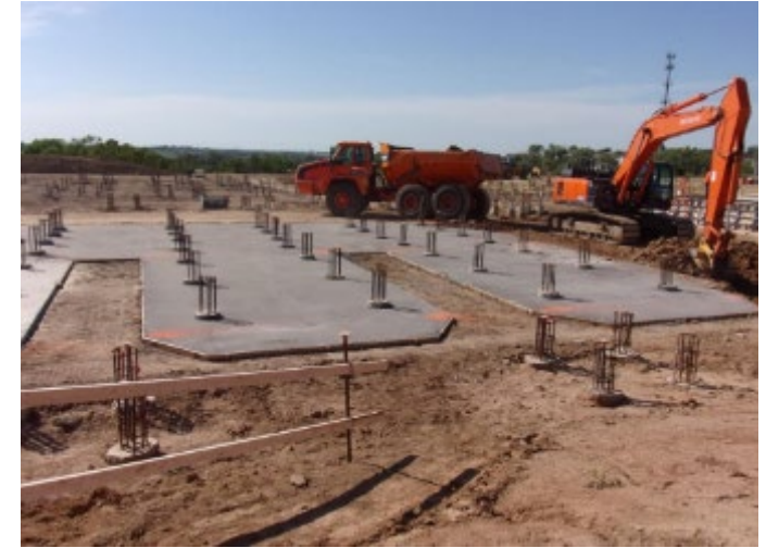
West Facing – Seal Slab Engines 4-6
