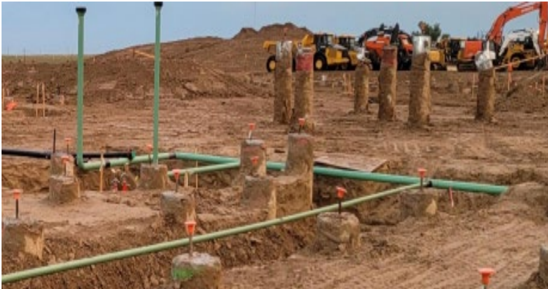
Facing Southwest – Unit 1 GTG Piping
