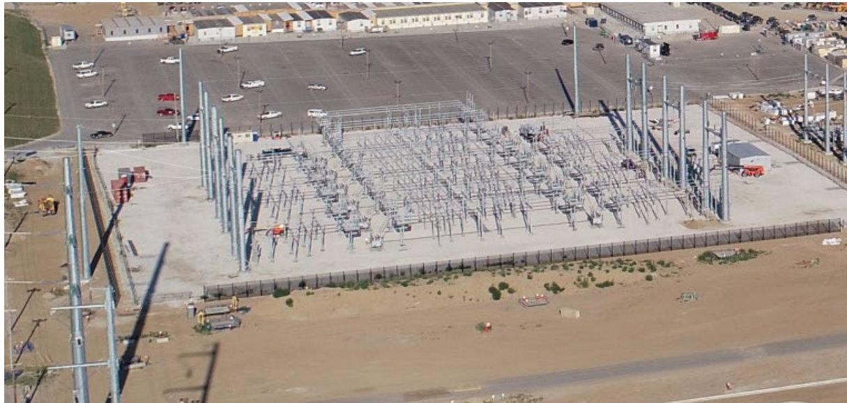
(144 th and Capehart Substation)
