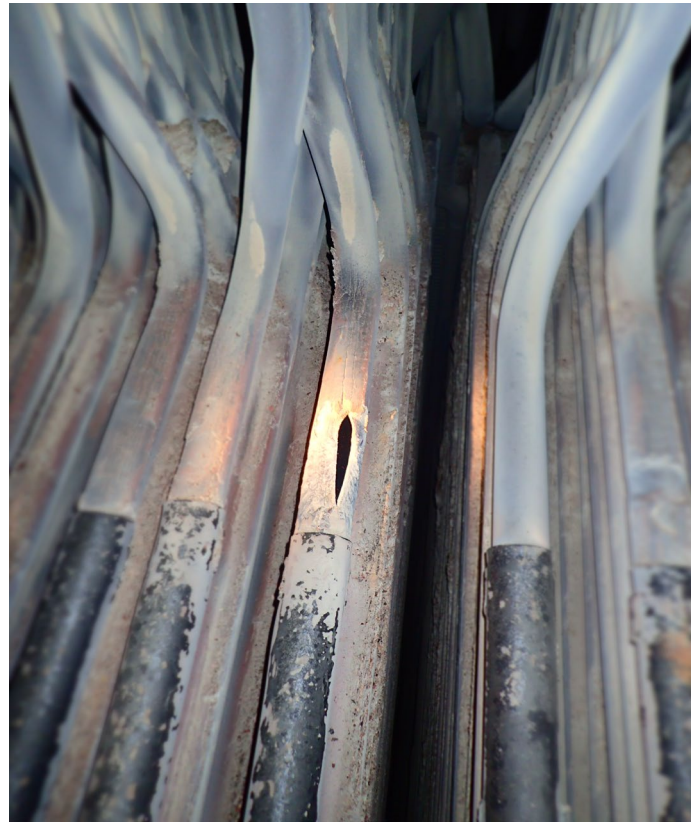
Reheat tube failures on NC2
