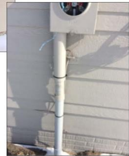
R-3 Expansion/slip riser setting is over two inches.
