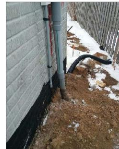
R-2 Vertical run not flush with the outside wall.
